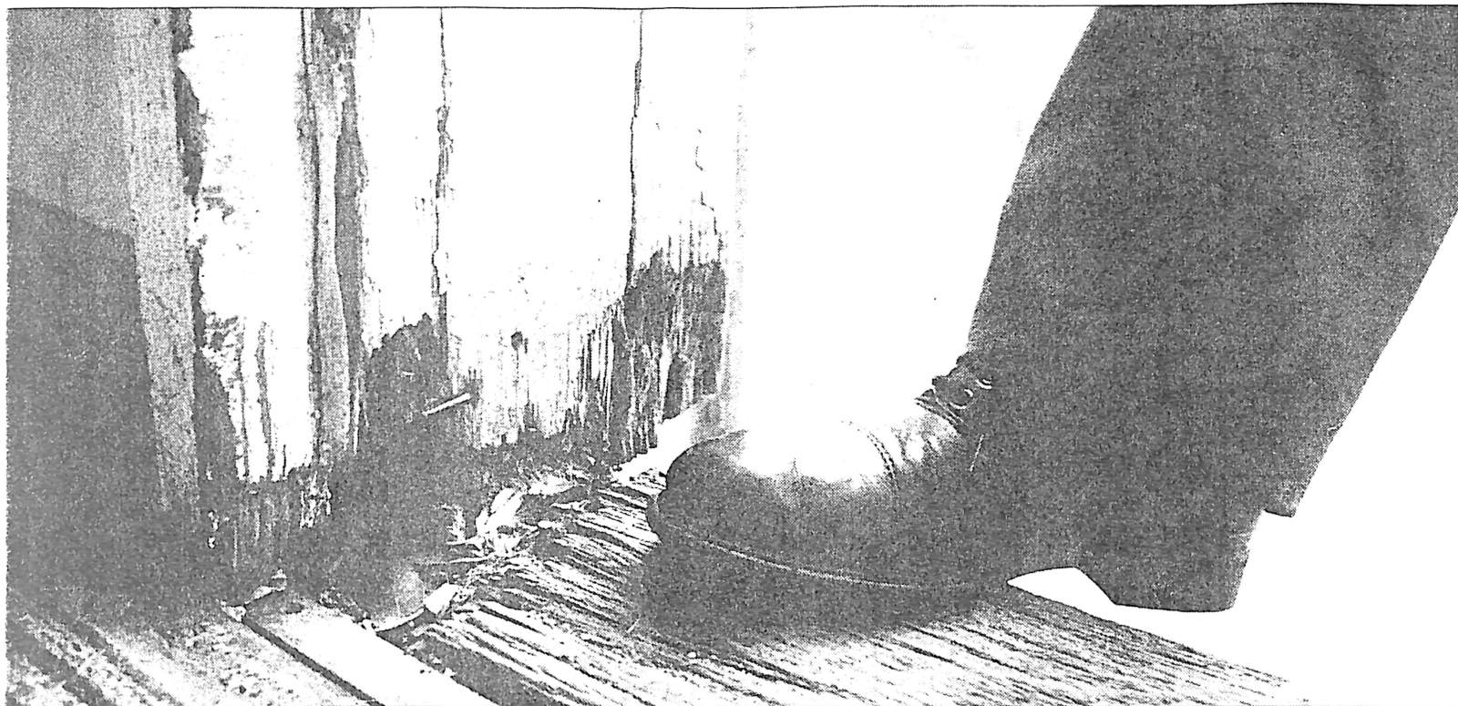
ing apart: steps outside the Ringwood Secondary College building which the school says desperately needs repair.
