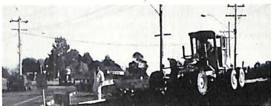
Spreading asphalt pavement material at intersection of Oban and Wonga Roads, Ringwood
