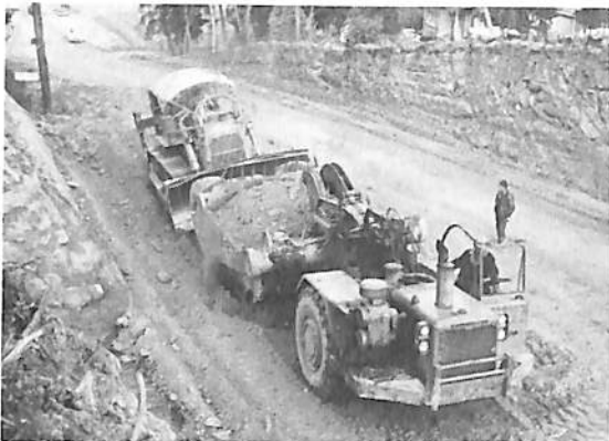
Excavation through hill for road works in Wonga Road south of Plymouth Road
