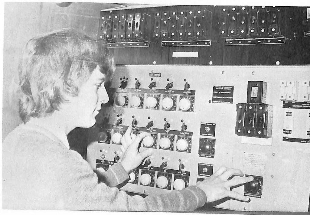
Mark Heyning at Hall switchboard.
