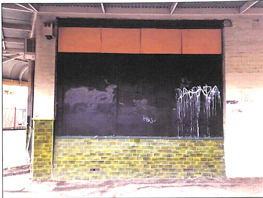
Figure 24 The shopfront and glazed dado on the west side of this Bedford Road façade, which is otherwise of pointed red brick now painted over.
