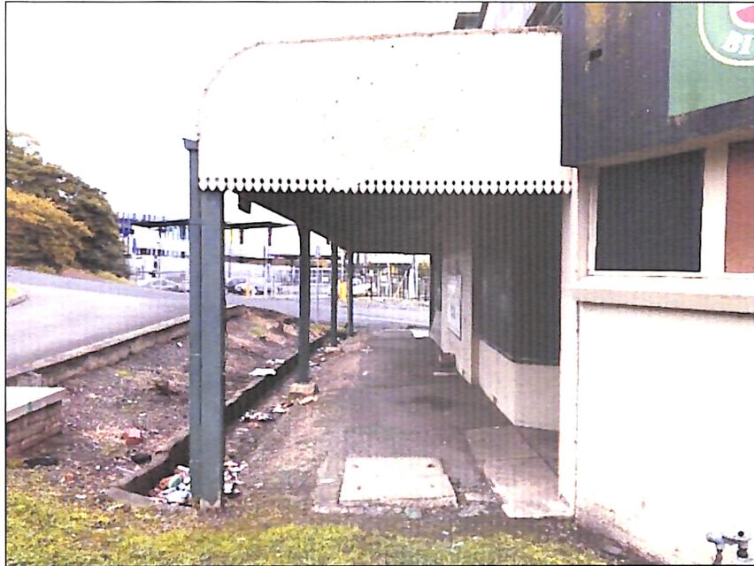
Figure 26 Side view of the east end of the reconstructed verandah along Bedford Street, showing the non-original bullnose profile and decorative timber trimming.
