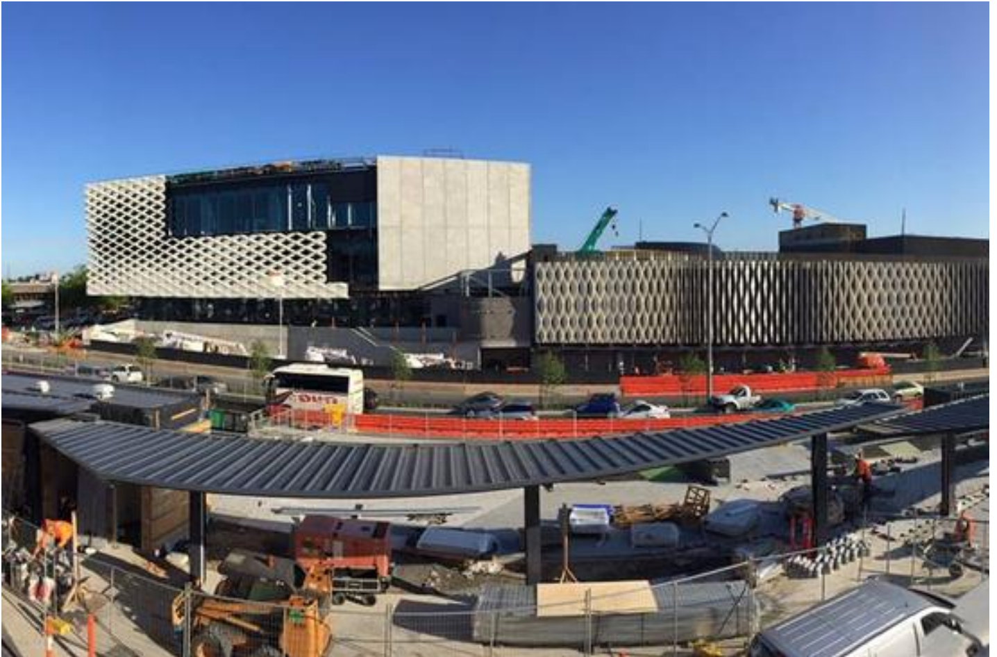
About 2000 people are working on the construction ahead of the opening on October 29.
