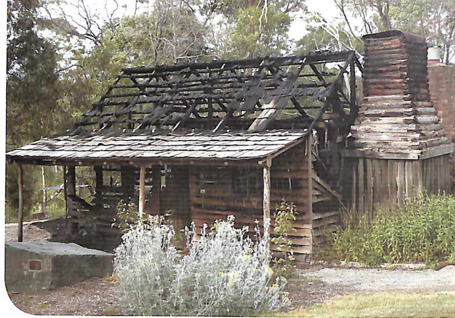
In 2009 the Maroondah Miners Cottage, a reproduction of one that stood at 367 Maroondah Highway, Ringwood in the 1880s, was burnt down following an arson attack.
