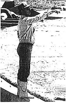
• At the cement face, Dr Dante Bini oversees the inflating of the binishell.
