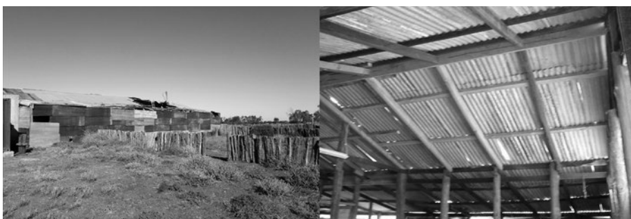
Figure 8. Nanya shearing shed showing Native Pine supports and repairs with treated pine. Source: M. Westbrooke January 2010.
