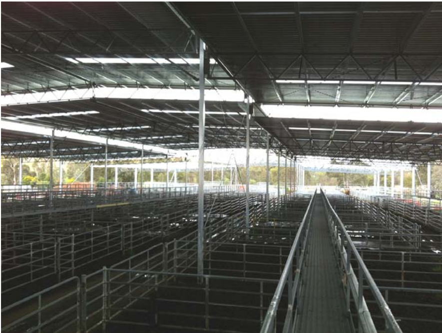
Photograph: Almost complete, the roofing of the Yea saleyards is progressing rapidly.
