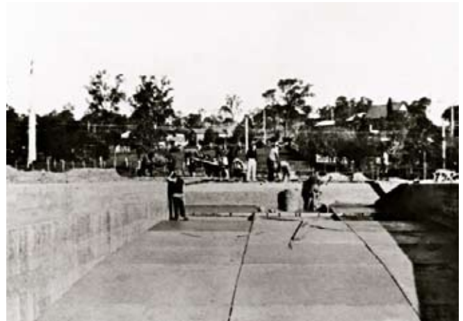
Work in progress on the Eltham Swimming Pool - 1933 Shire of Eltham Pioneers Photograph Collection
