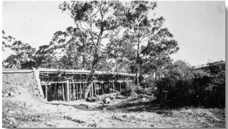
Construction of the new concrete bridge c. May 1926 Photograph - *EDHS SEPP collection
