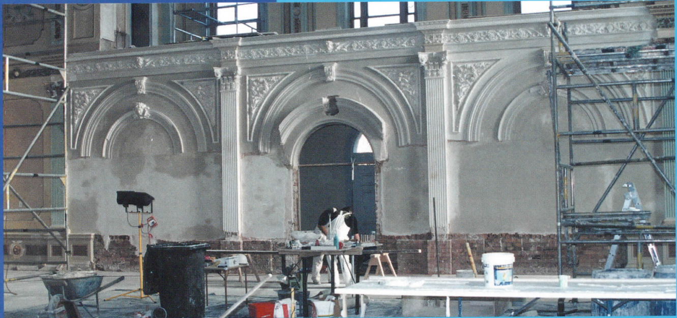
The reinstatement of the original balcony involved the erection of the supporting brick wall removed in 1926. The wall was modelled on photographic evidence.
