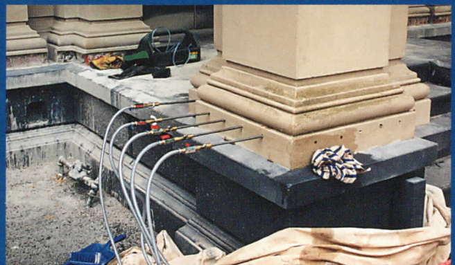
The damp proof course was chemically injected in all basement walls and around the perimeter of the building.
