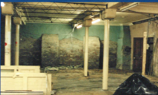
An issue of rising damp had to be addressed before any interior works could start. The first stage of the project started in the basement and involved the installation of a damp proof course.
