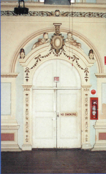
The decorative elements of the main hall had suffered considerable damage through wear and tear as well as inappropriate installation of services.
