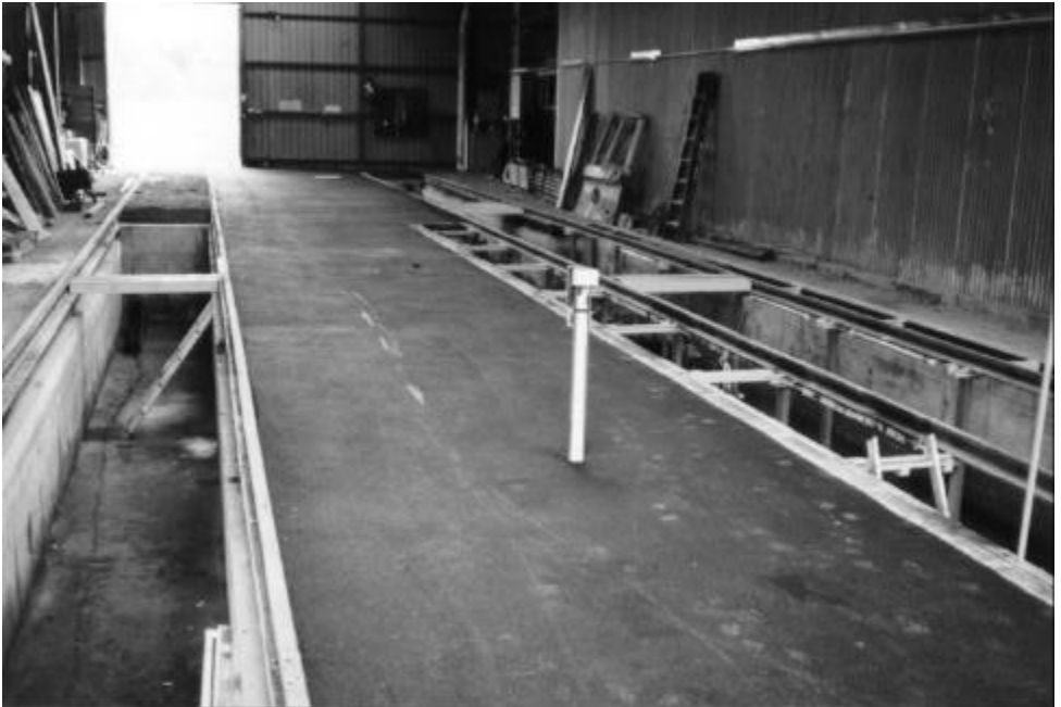
Photographed shortly after completion is the new hot mixed surface in the depot between No. 4 and 5 roads on Monday 1 September 1997. Photo: Warren Doubleday
