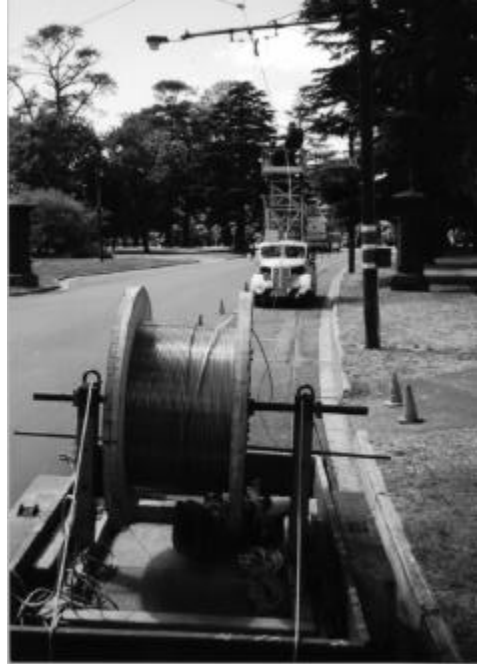
The new overhead cable has reached Carlton St, but awaits more poles before heading towards Sturt St. West and the City.
