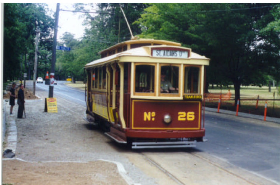
Tram 26 being driven by Anita Bagley passes the roadwork site showing the new kerb and channeling at our Depot Junction tram stop. The tram track had been surfaced when this photo was taken on 12 December 1998, but the new roadway around the stop itself was not completed until about a month later. Photo: Warren Doubleday
