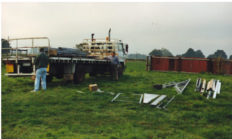
Offloading the components for the new sheds at Bungaree, 4.10.1999. Photo Carolyn Dean
