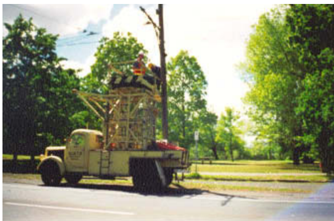
Mark McKay and Warren Doubleday take down the signal boxes in Wendouree parade for rebuilding. Photo Clare Johnson
