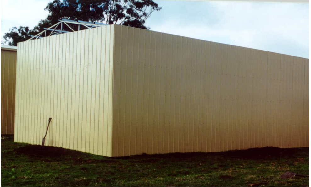
The wall cladding of the second of the two sheds is completed, with the first behind it. Photo Carolyn Dean – 6 May 2000.
