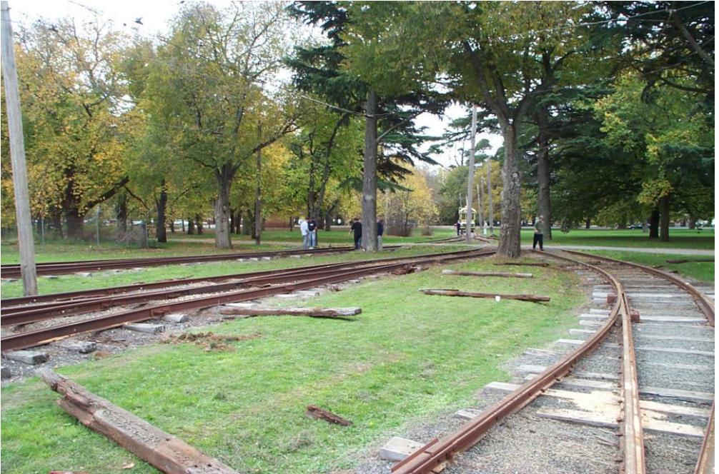
The scene at the depot on Sat. May 12 during the replacement of sleepers in the Depot fan area. Photo Warren Doubleday
