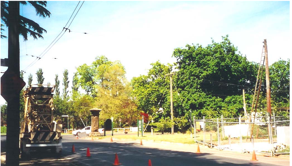
Below: The former span wire pole standing at the entrance footpath to the Ex-Prisoner Of War Memorial. Monday 17/11/03. BOTH PHOTOS RICHARD GILBERT
