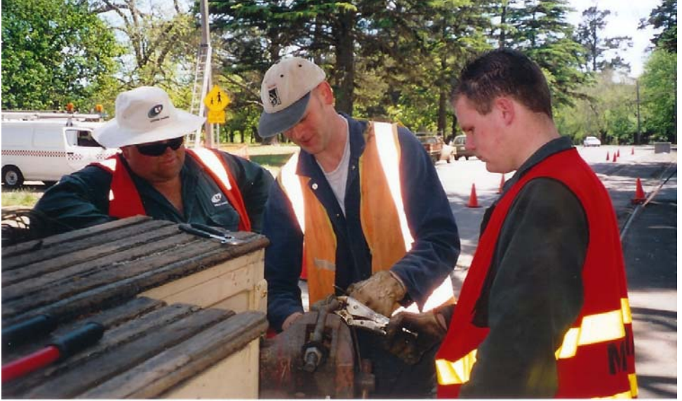
Above: Andrew Cox, Garry Wood and Alastair Reither making up an overhead component for the span wire relocation.
