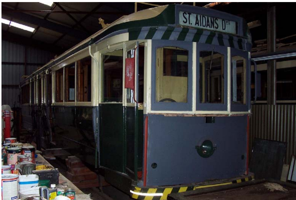
No 40 is starting to look like a tram again, with the head lights fitted to the end panels and the first of the green colour applied. 6 August 2005.
