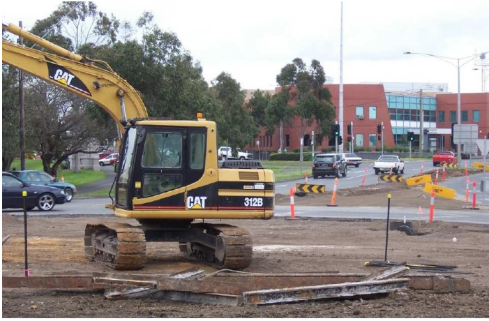
Left: Rail being removed from the intersection of Malop and Gheringhap Street, Geelong Photo: Richard Gilbert
