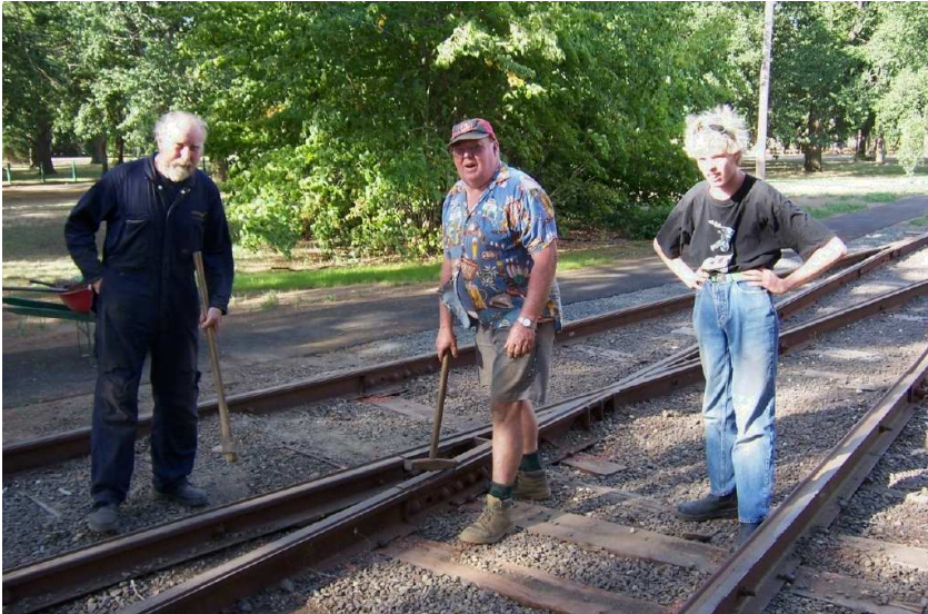
Dave Macartney, Phillip Work and Daniel Edwards take a moment from hammering dog spikes into the new sleepers they have inserted into the access track.
