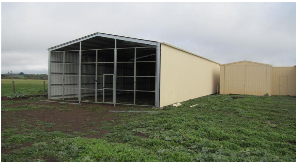
The new storage shed at Bungaree. The doors have now been sheeted.
