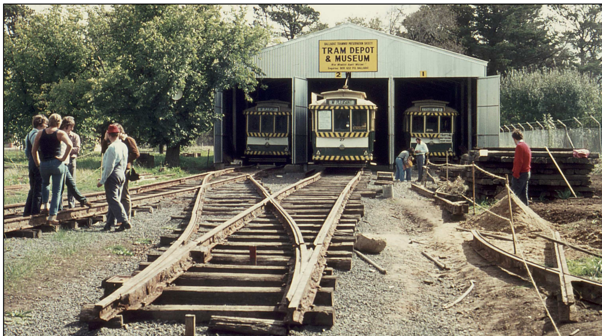
Above: The depot fan circa late February 1973. The track under No 27, the first to be laid has never needed repair. The workers standing on the left include Geoff Cargeeg, Bill Kingsley, Stuart Lodington and Gavin Young Photo: Peter Winspur
