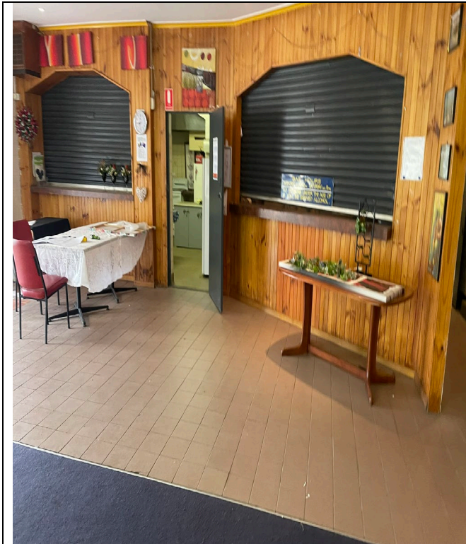
Mixed hard and soft covering to slab on ground in clubroom area generally in acceptable condition.
