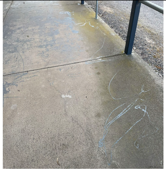
Some general shrinkage cracking to slab area.
