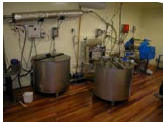
Extracting plant – note polished timber floor
