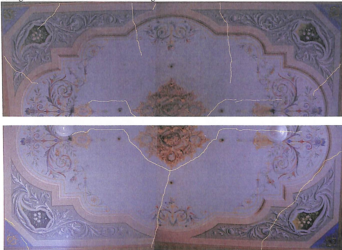
Figure 5 Cracking to the plaster in G4. The yellow lines mark the extent of cracks in January 2004.
