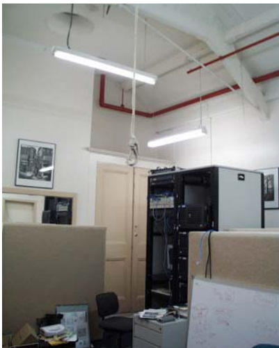
3. Server room G.11, south wing
