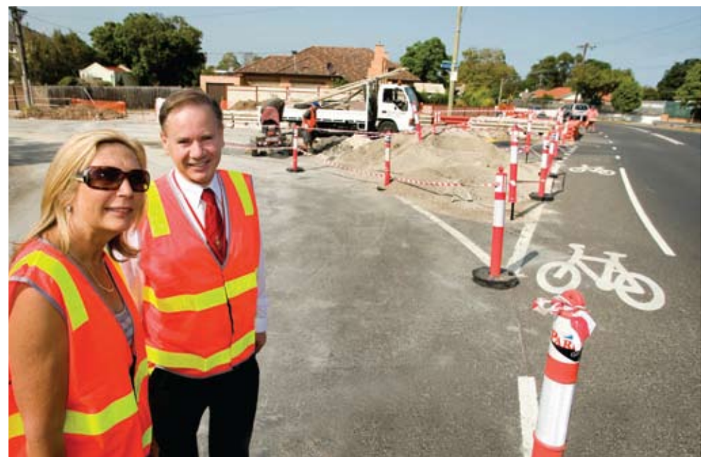
Glen Eira Mayor Cr Helen Whiteside and Bayside City Council Mayor Cr James Long at the site of the new roundabout. Photo: Bernie Bickerton.
