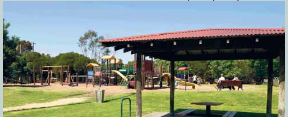
Works have commenced on the redevelopment of the play space at Murrumbeena Park.
