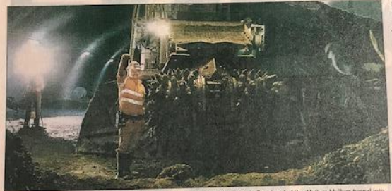
At last: EastLink tunnel concreter Nigel Daly takes the first steps from the Springvale Road end of the Mullum Mullum tunnel into the Deep Creek Road section. Picture: Julie Boyer
