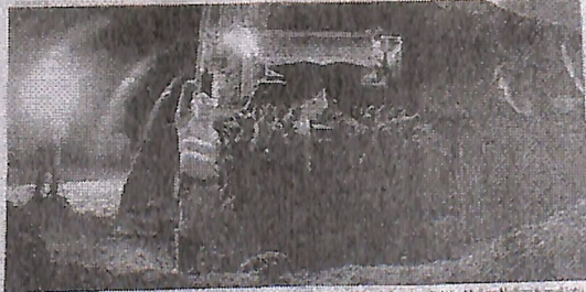
At least 100 miles of tunneling will be done to take the first steps from the Springfield Road end of the Madras-Melrose tunnel to the Dale Creek Road section.
