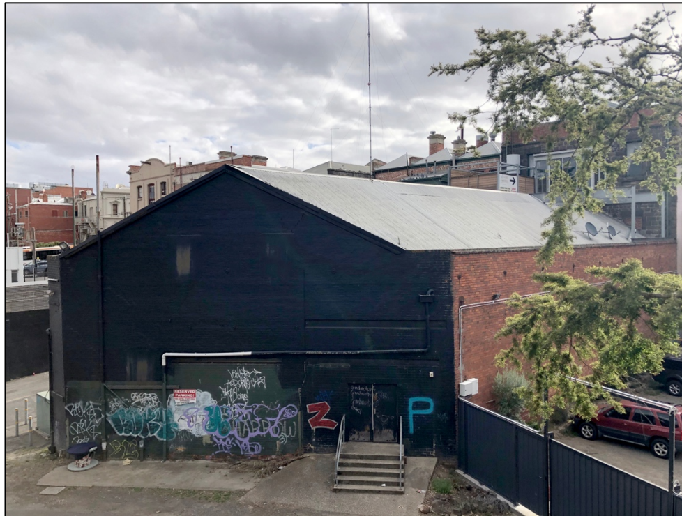
Figure 10 The early twentieth century gabled brick addition to the rear of the former warehouse at 122 Lydiard Street.
