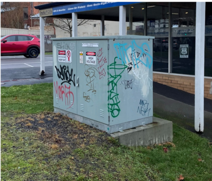
Figure 7 Authority substation close up
