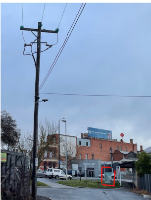
Figure 5 Pole on corner of Bradbys Ln/Porter St and substation in background
