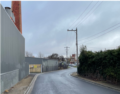
Figure 4 Existing authority electrical infrastructure in Porter Street
