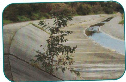
River Red Gum clinging to life in a crack in the concrete channel
