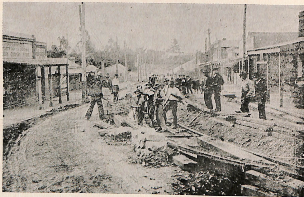
New rails for the electric trams replace the old steam tram track at Long Gully.
