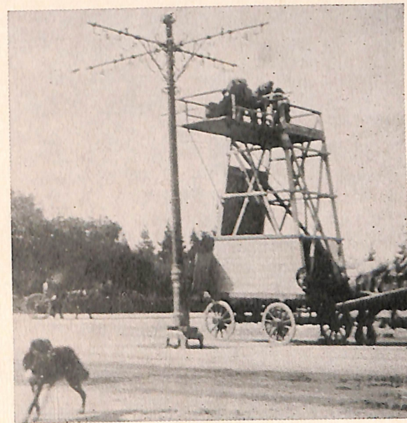
Aided by a horse drawn tower wagon, workmen erect overhead wires on the four bracket arm pole at the hub of the system.
