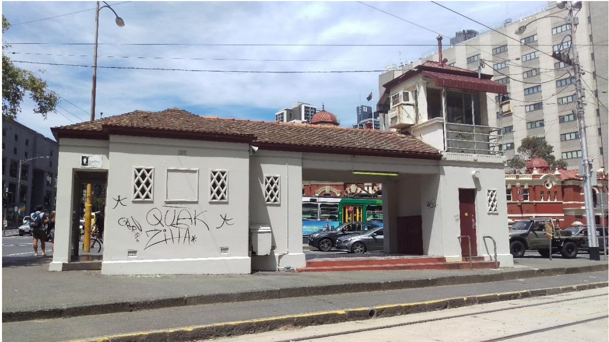
Figure 9: Graffiti on the face of the Tramway Shelter. Source: Y Gaoulii, taken 3 December 2016
