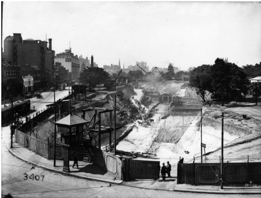
Figure 8: The signal box at Elizabeth and Liverpool Streets (foreground) during the construction of Museum Station in Sydney.
