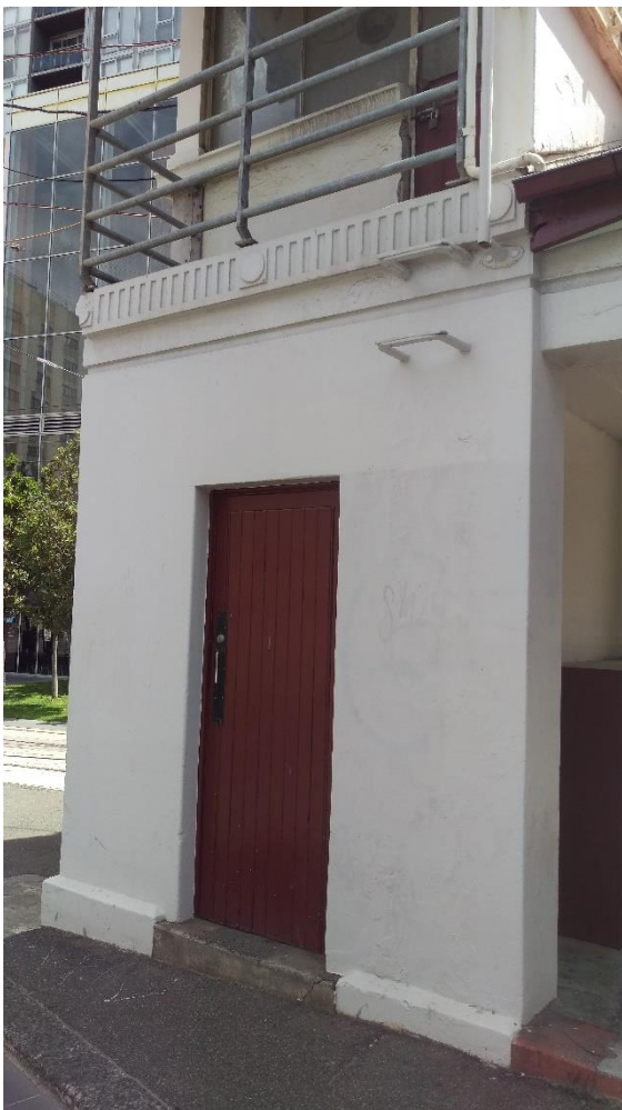
Figure 6: The eastern face of the building at the southern end, showing the remaining step rungs. Source: Y Gaouil, taken 3 December 2016
