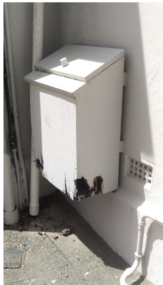
Figure 7: The damaged wooden box. Source: Y Gaouil, taken 3 December 2016
