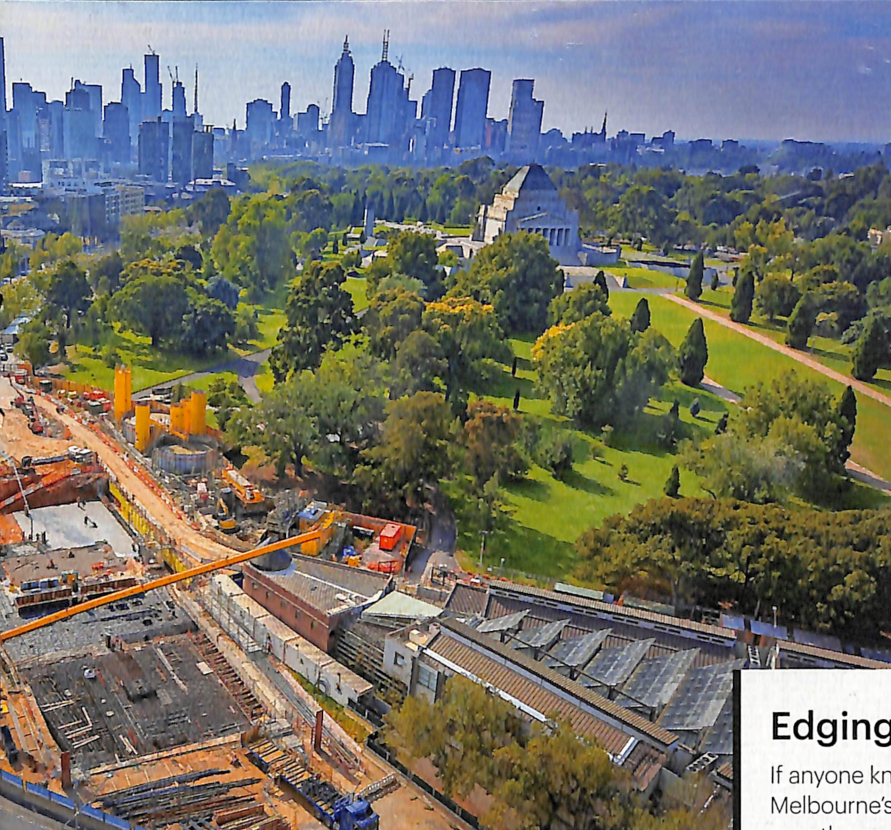
(From left) Electric tramway construction at the intersection of St Kilda and Domain Roads around 1925; building the Metro Tunnel Project's Anzac Station at the same intersection in 2019.
