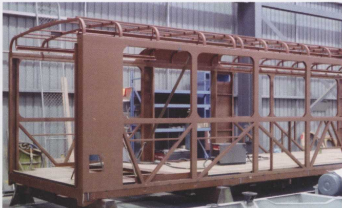
The bare shell of one half of a B-class articulated tram under construction at Comeng Dandenong in April 1983.
