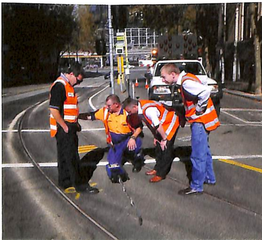
LEFT: Yarra Trams engineering staff are working with Voestalpine on constant development of new products and processes.
