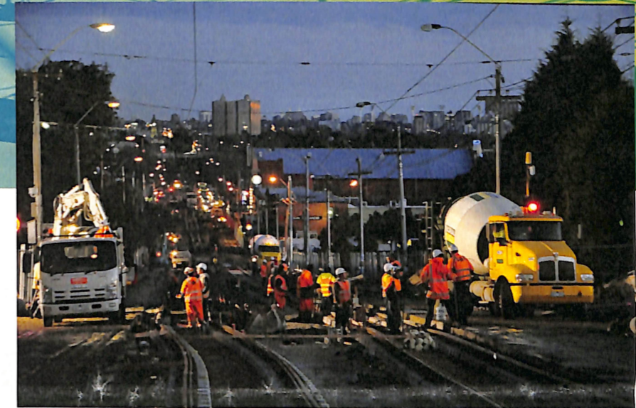
RIGHT: Works along High Street continued 24 hours a day for seven days until the big job was finished.
