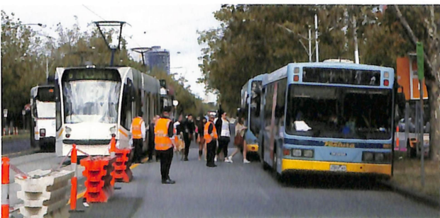
TOP: Works continued 24 hours despite the weather. ABOVE: Staff assist on a tram/bus connection.
