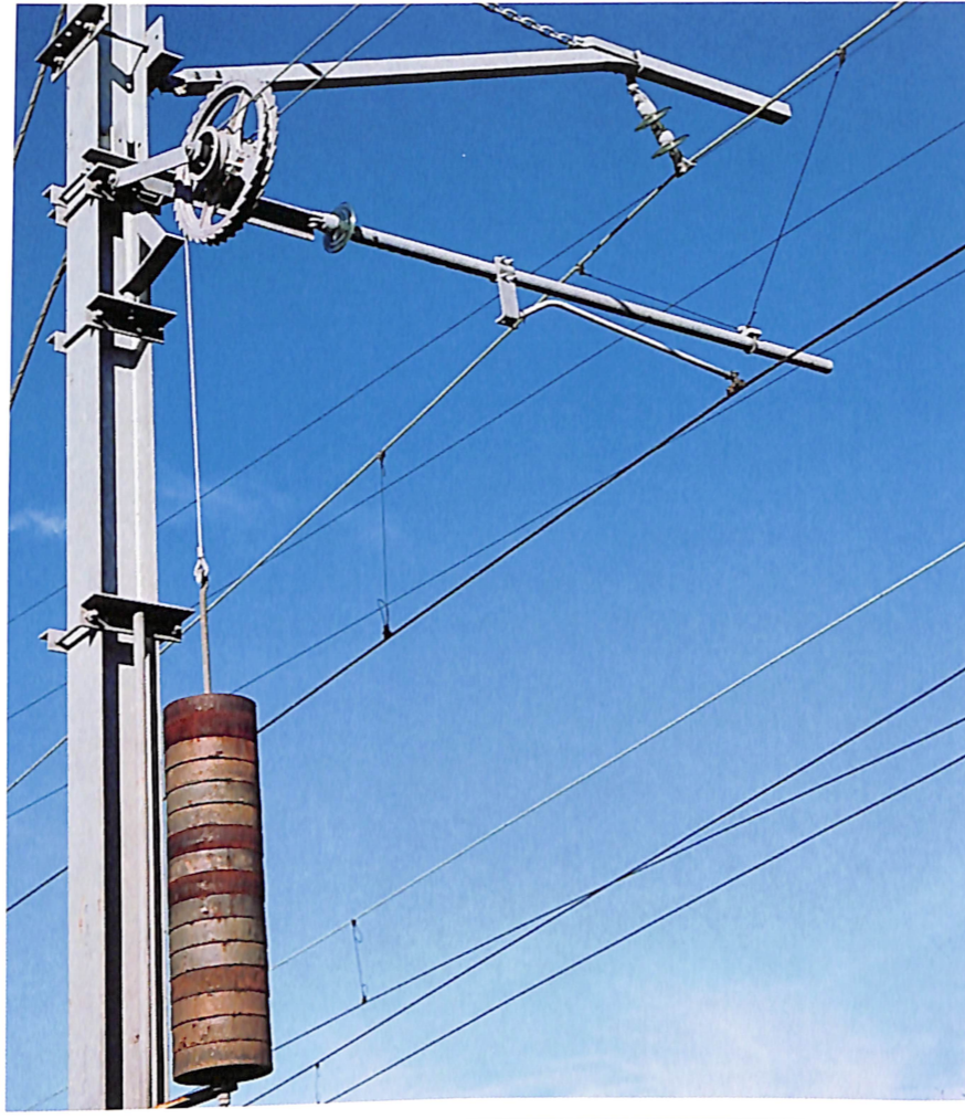
Boom cantilever & contact wire balance weight assembly
