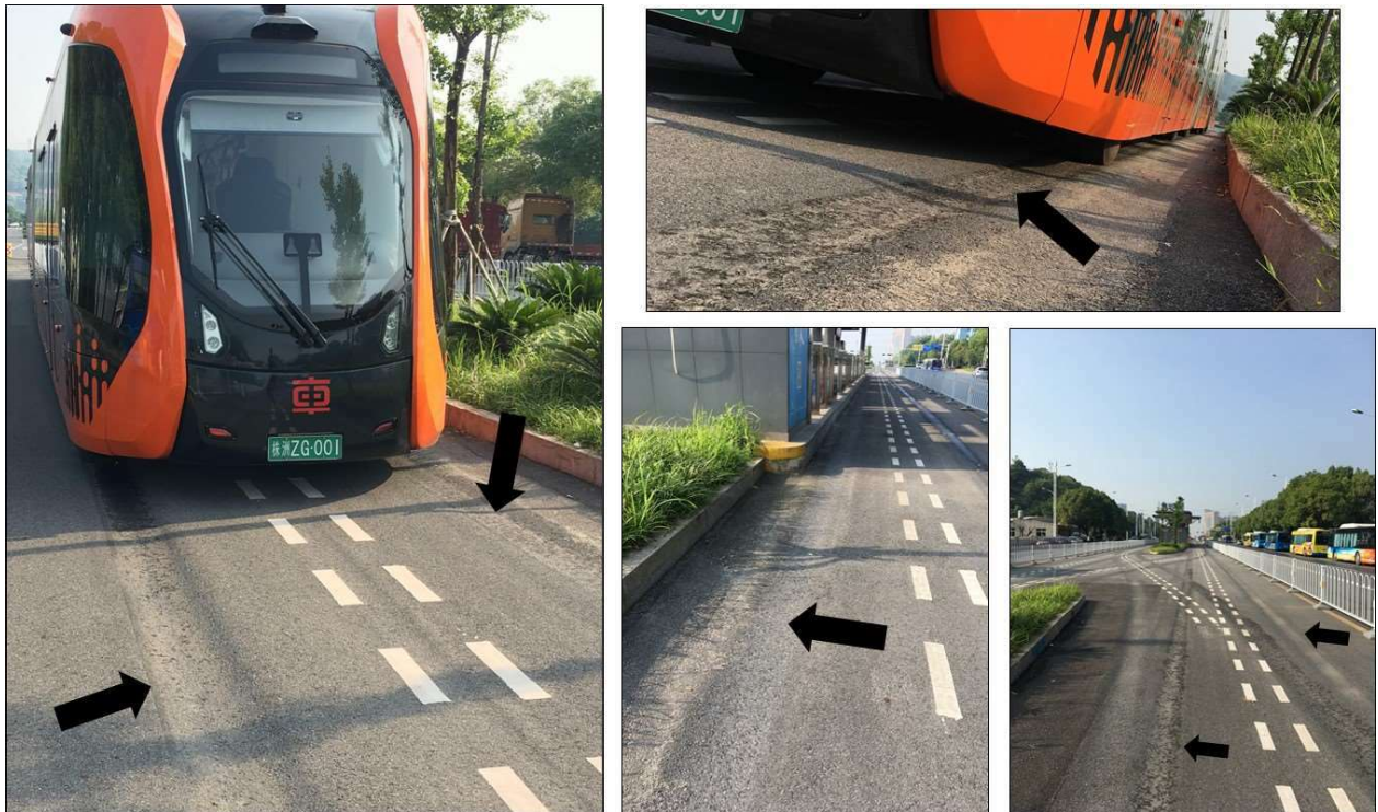
Figure 1: Photographs of Road Pavement ‘Rutting’ – Zhuzhou China Trackless Tram
