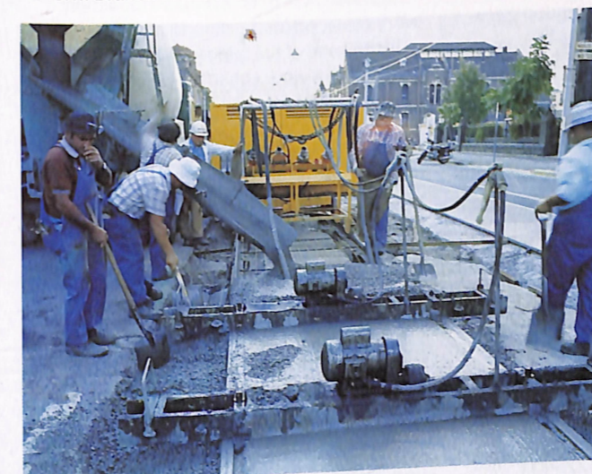
Track upgrading on a section of line at Windsor. About 70 percent of the tram network has now been upgraded with concrete to surface base.
