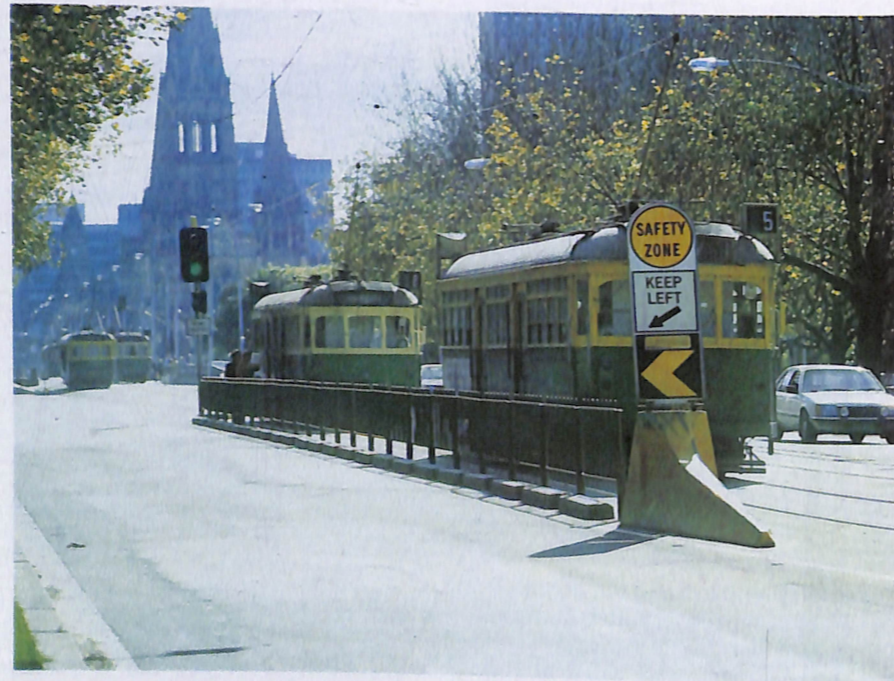
The installation of tram safety zones around the network forms an important part of the activities of Civil Branch.
