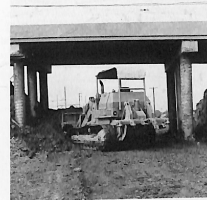
Work being carried out on a tunnel under the rail line will provide access to new parking areas.
