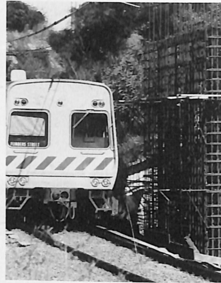
A Flinders Street bound train passes part of the structure which will form a new bridge at Brown Street, Heidelberg.
