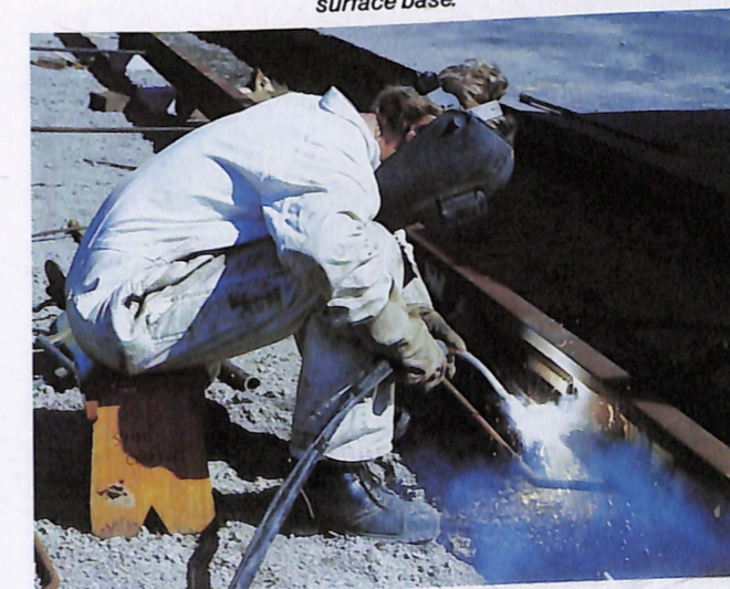
Steve Chambers welds a track joint on a section of tram line in Burke Road, a busy section of the network.
