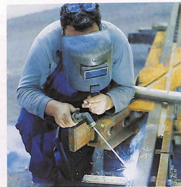
Rail fabrication for use in the tram network forms an important function at Civil Branch. Here Michele Giannetta works on a section of rail at the South Melbourne yards.
