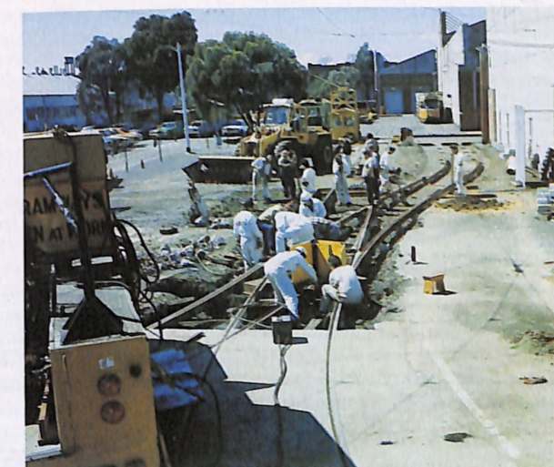
Track reconstruction at Preston Workshops is being carried out to accommodate delivery of the LRVs due to enter extensive service shortly. Gangs from Civil Branch are also involved in this project.
