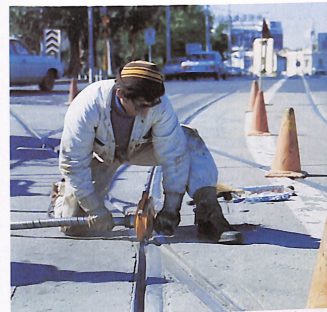
Peter Kargas makes some important repairs to track on a section of the tram network. The biggest percentage of work carried out by Civil Branch relates to track maintenance and construction.
