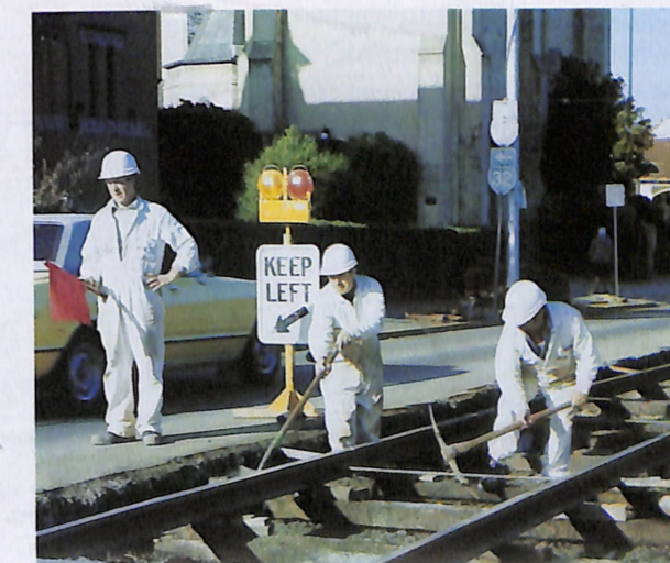
Working on a section of track in preparation for upgrading work. From left to right: P. Lombardi, S. Luci. The flagman controls traffic flow.
