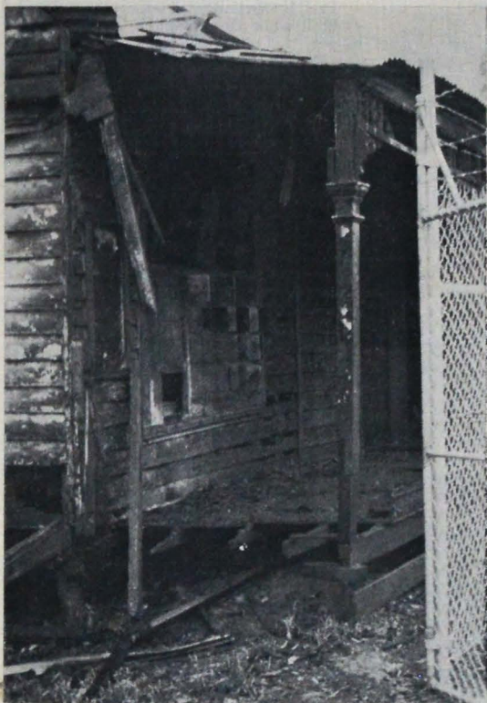
The charred remains of the front verandah section following the tragic fire.
