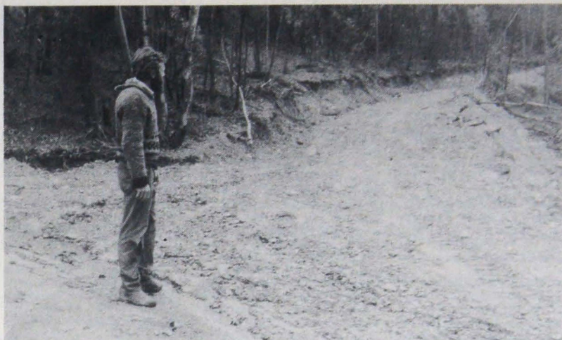
Doug Seymour of the WEL looks over the new road bulldozed from Wyuna Road.
