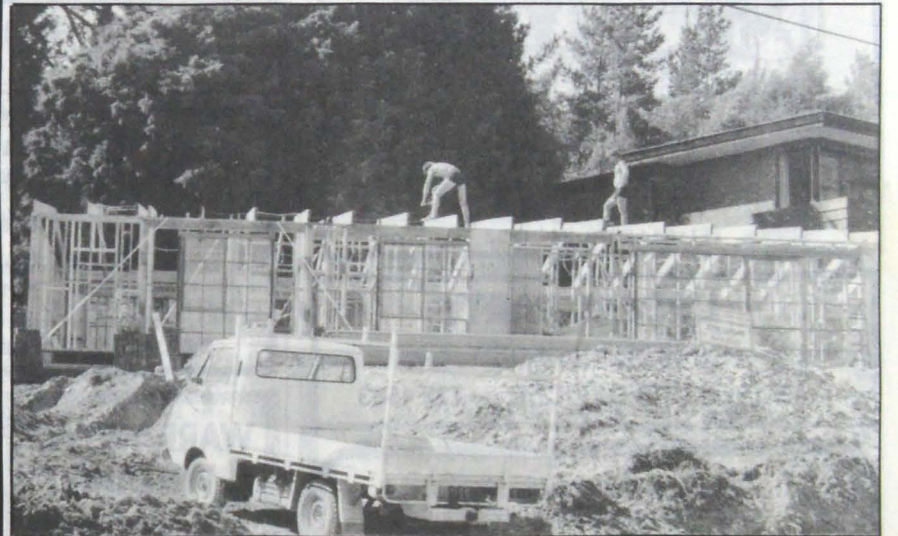
Work is proceeding apace on the controversial new house in Anderson Street, being built under an 'as of right, dual occupancy' permit.
