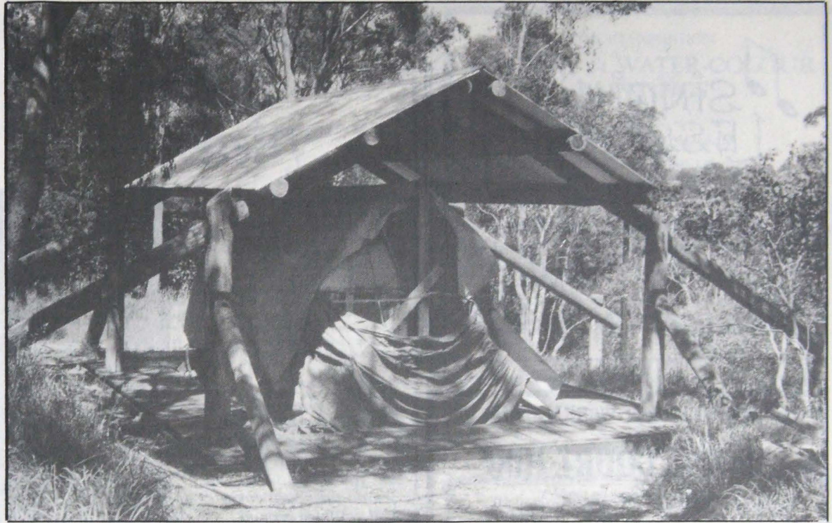
This sturdy roof, built by National Trust tradesmen, now shelters the hut.
