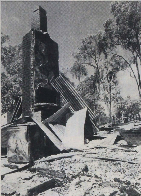
All that remained of Victoria's historic first youth hostel at Pound Bend following the 1991 bushfires.
